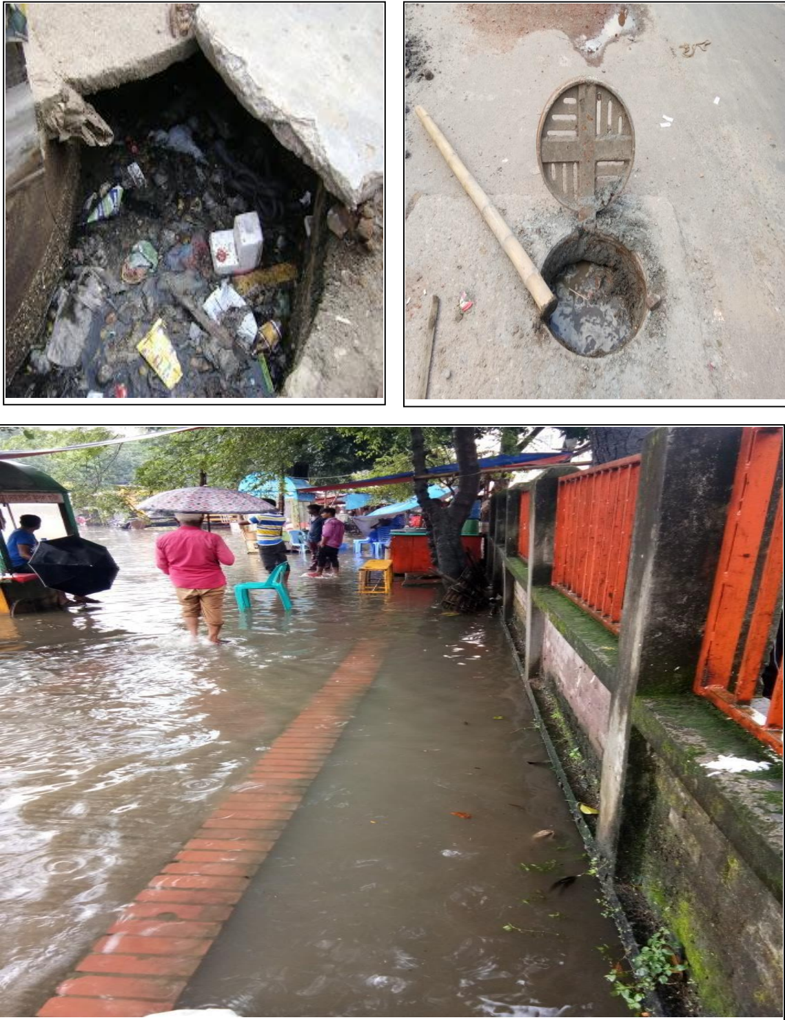
Figure 2: Blocked Drains and Manhole at Dhanmondi residential area
